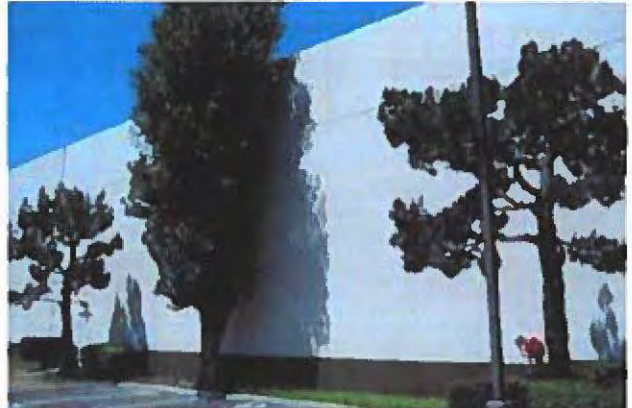
View of the portion of the south wall at the TY North America space.
